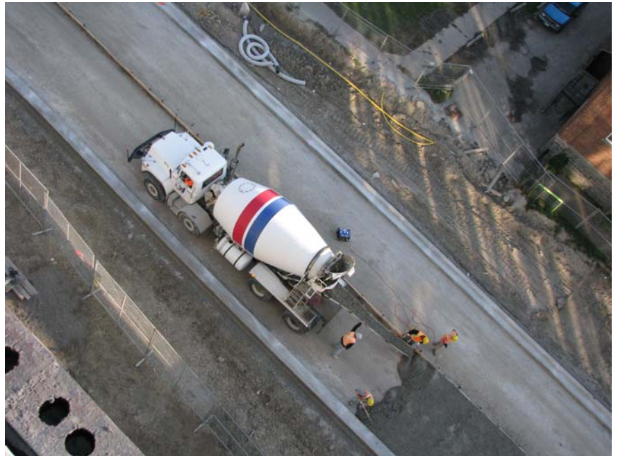
Site staff pour the concrete for the Sackville Street extension on October 18, 2008.
